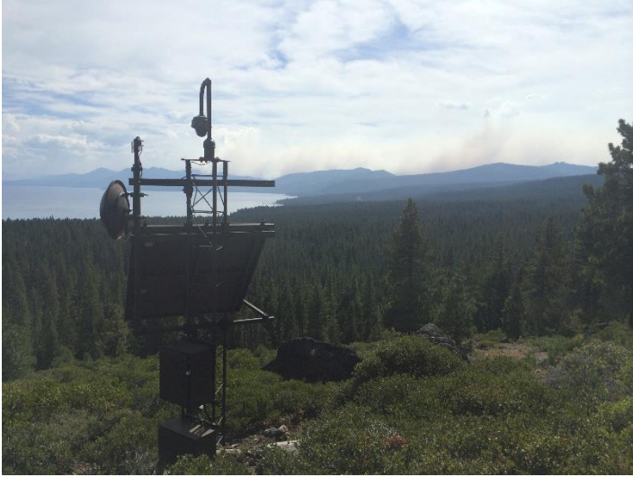
Figure 1. IOT EEW and ALERTWildfire site at Dollar Point, California.
